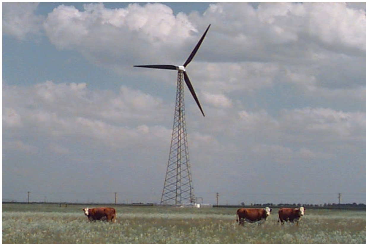
Pictured above is one of the two 750 kW wind turbines near Springview
